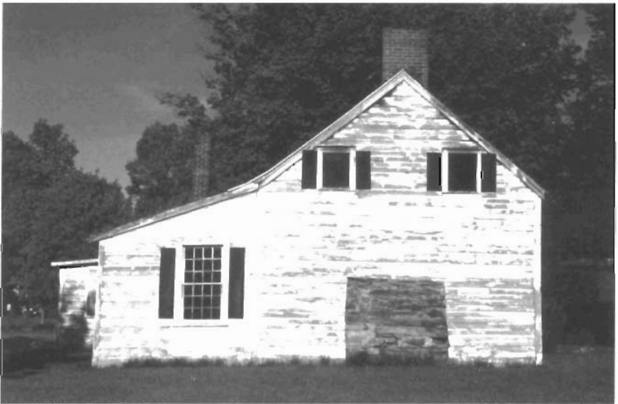
West Elevation. Log section (c. 1776) under gable roof; lean-to added c. 1910. Note stone back of fireplace exposed on exterior with bulge due to collapsed foundation.
