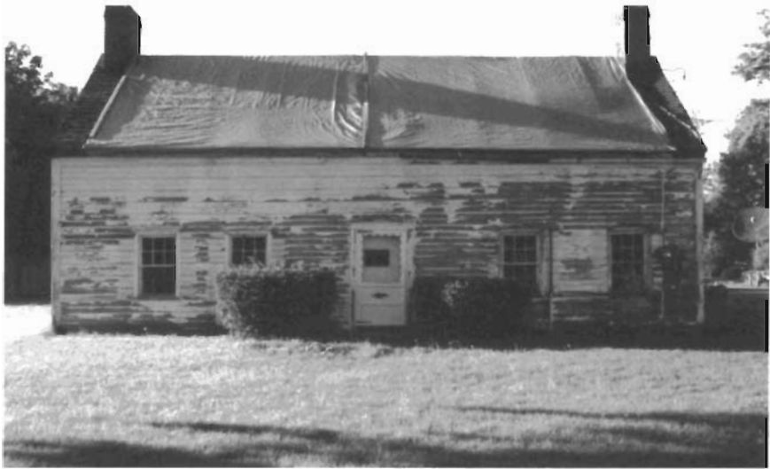
South Elevation. Original one-room log hut (c. 1776) left of door; log addition (c. 1776-1778) on right; window sash installed c. 1820; wall rebuilt and siding added c. 1888. Note failed asphalt shingles roof.
