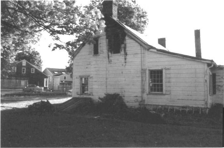
East Elevation. Log addition on left under gable (c. 1776-1778) with rebuilt chimney (c. 1820); lean-to (c. 1910) on right. Note fire damage around window outside the room where the arson took place.
